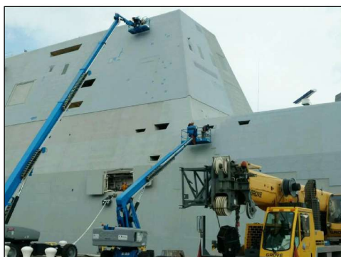
(Top right) Scale embedded on steel flange with its before and after weight related to rust treatment. (Photo Credit: Nuclear Engineering Training Laboratory, University of Texas) (At right) USS Zumwalt during cleaning. Note the left side of the ship after cleaning with EPDI's Enviroklean.
